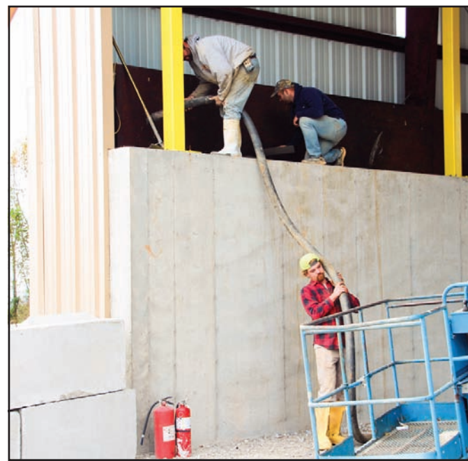
Workers pumping concrete into the new walls erected inside the commercial dumping shed at the Transfer Station last week. Photo by Shawn Jarrard
