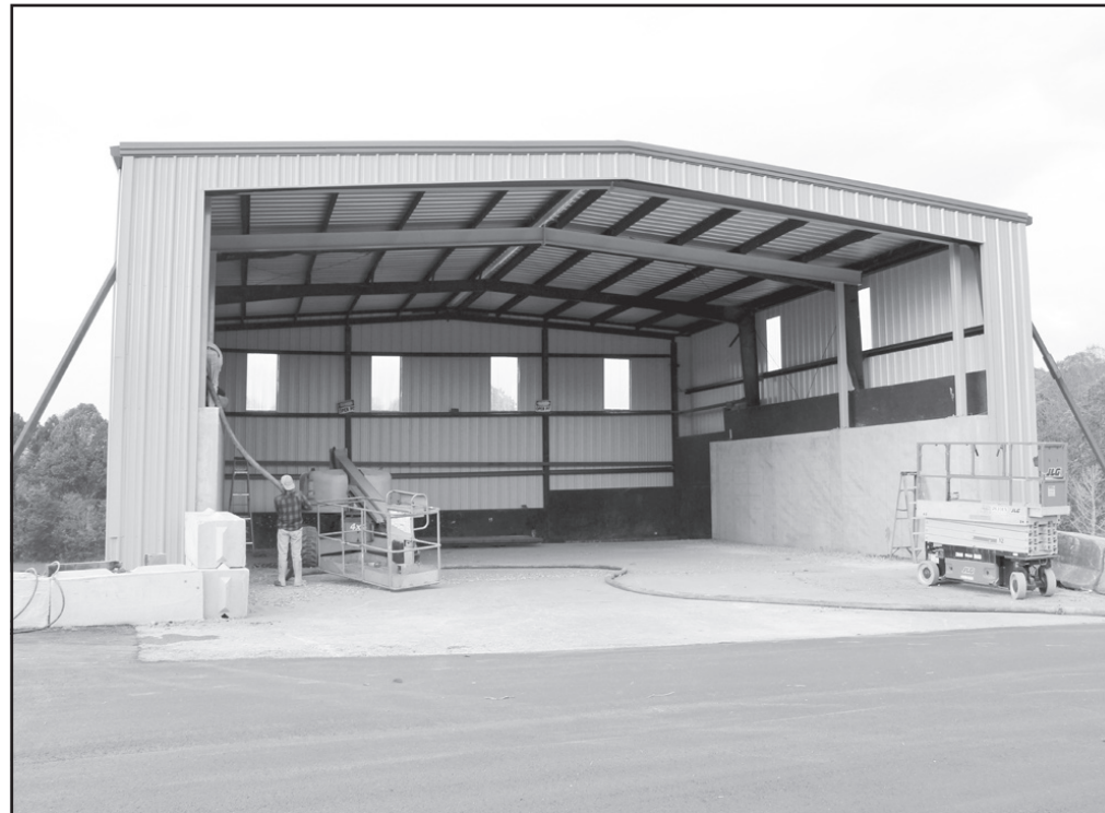
The big shed at the Transfer Station has gotten a facelift – and important safety improvements, too – in preparation for re-opening later this month. Photo by Shawn Jarrard
